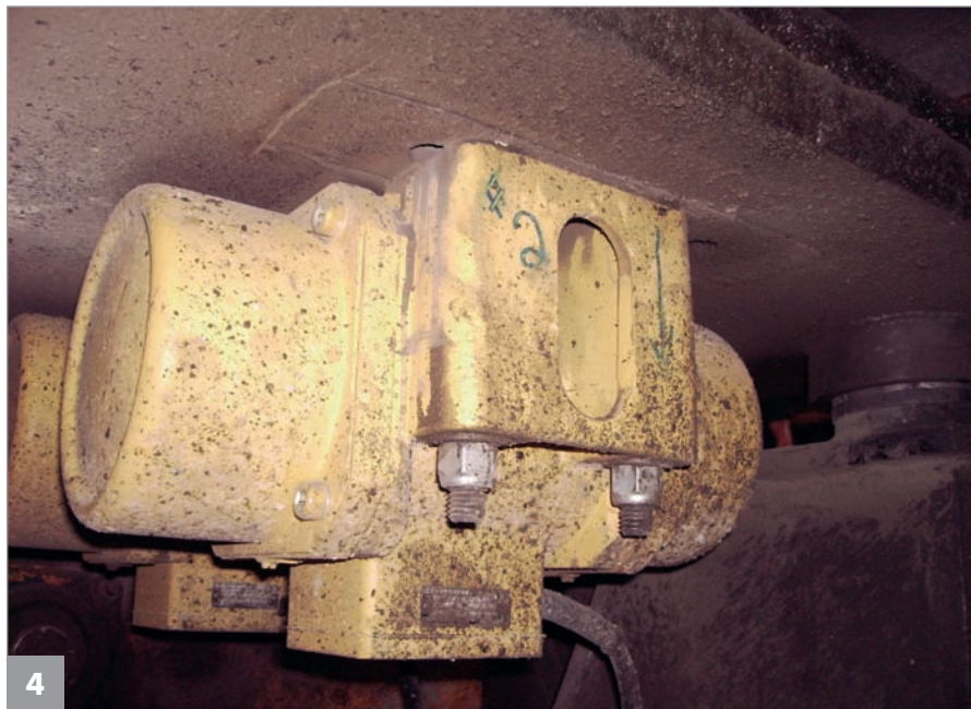
4 Vertical vectored vibration caused by two external vibrators model Bosch 18120.
