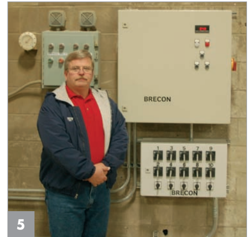
5 Randy Molin, facility manager, next to the new control unit.
