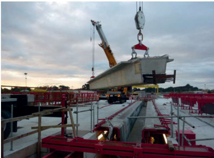
The project is being built by an alliance made up of the NZ Transport Agency and several specialized planning and construction companies.
