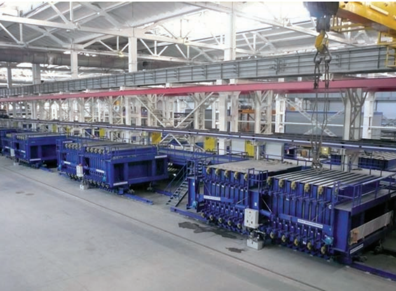
Fig. 2: A second row of four battery formworks runs parallel to the first row. The control equipment for the vibration is installed 'back to back' and has identical functions. The radio remote controllers are isolated from each other, however.
