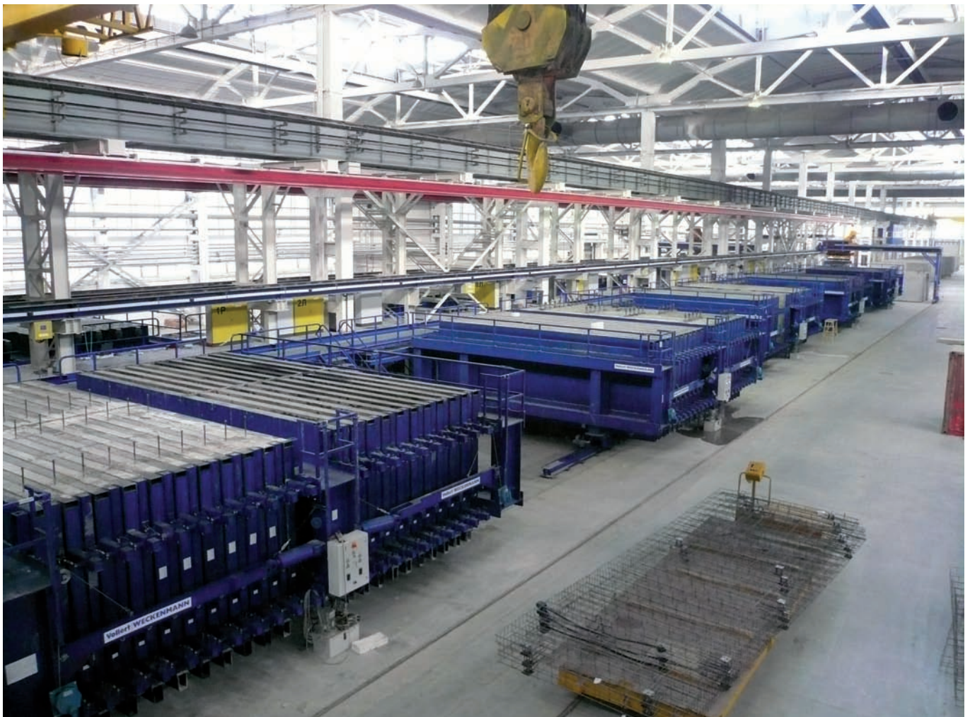
Fig. 1: The control equipment for the vibration of five battery formworks with almost 500 vibrators is installed on a railing at a height of 4 metres. All five control units can mutually replace each other without switching over (redundancy).
