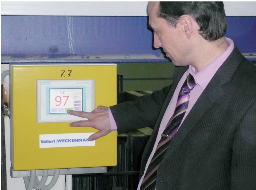
Fig. 8: Project manager Alexander D. Jaroshenko (DSK Blok) operates the vibration compaction via one of the new Brecon touch panels.
