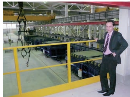
Fig. 10: The project manager Alexander D. Jaroshenko from DSK Blok is pleased with the clean, tidy installation
