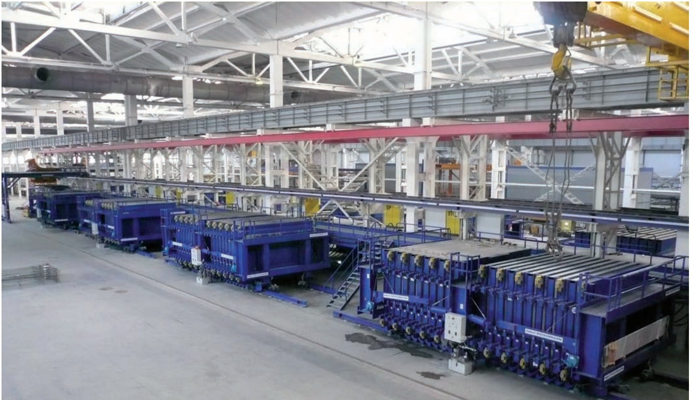
Fig. 2: A second row of four battery formworks runs parallel to the first row. The control equipment for the vibration is installed 'back to back' and has identical functions. The radio remote controllers are isolated from each other, however.
